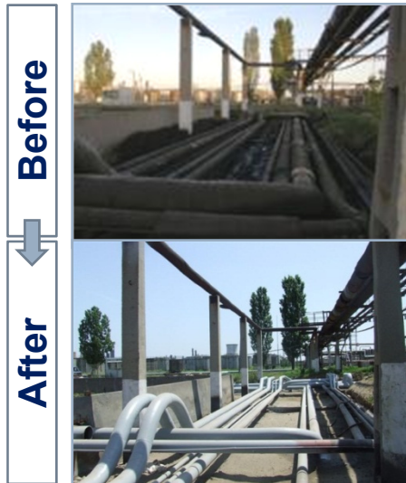
Picture: Sleeper road inside refinery before/after removal of unused pipes and renewal
