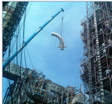
Picture: 52 inch transfer line change from 2x 24 inch; prior to CDU revamp
